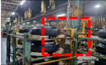
G/T carts stacked in front of fire hydrant
