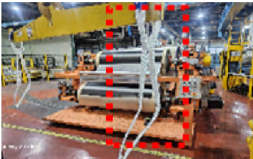
Sling belt replaced
