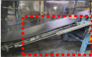
Protective railing dislodged
